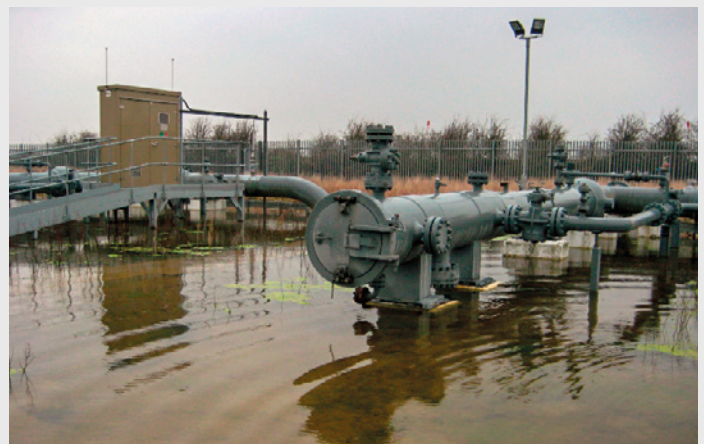
Figure 6.4: Flooding at the Gravesend Thames South above ground installation in 2013
