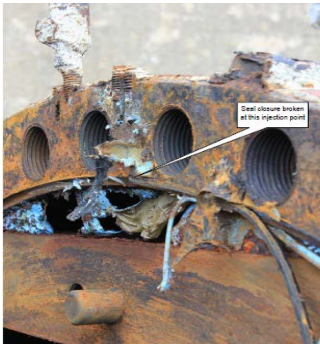
Picture showing failure of internal O-ring in valve closure and attempts to inject sealant into valve to repair leak.
