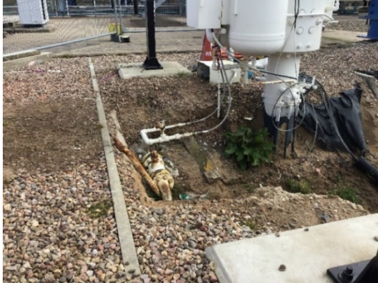
Figure 44: Corrosion and ground movement threats to Actuators
