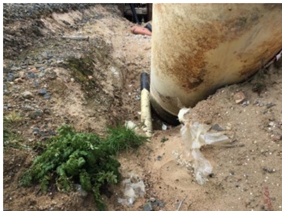
Figure 6: Actuating pipe clashing with main gas line due to ground movement
