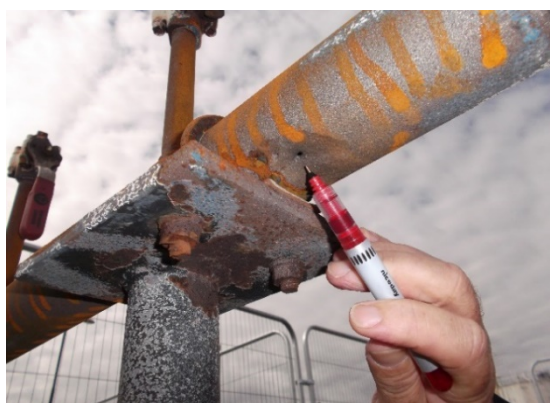
Figure 10: Through wall corrosion leading to pinhole leak requiring replacement
