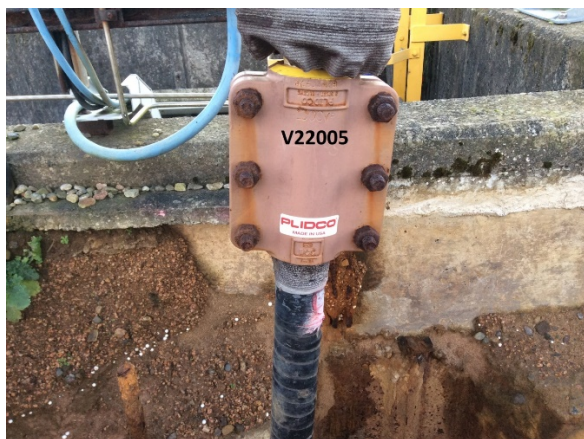
Figure 11: Temporary Plidco Clamp on Actuating pipework riser
