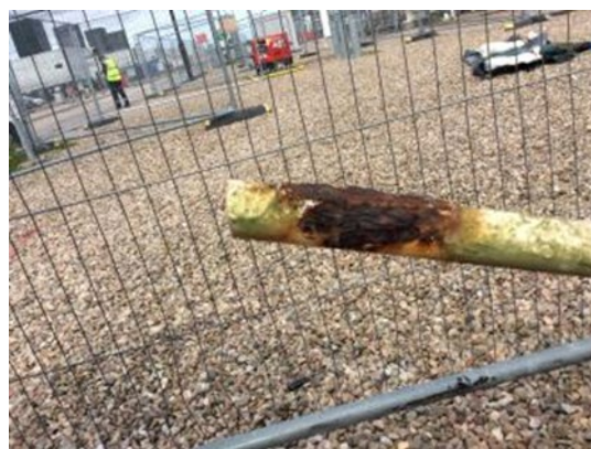
Figure 9: Through wall corrosion requiring replacement to continue operation
