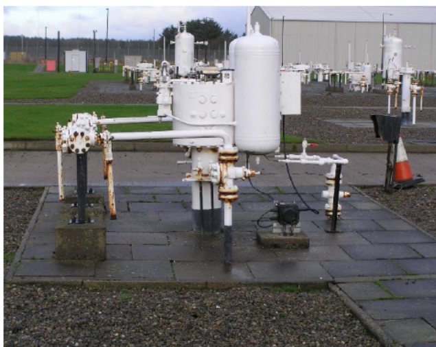
Figure 3: Typical gas-powered Actuator at St Fergus terminal
