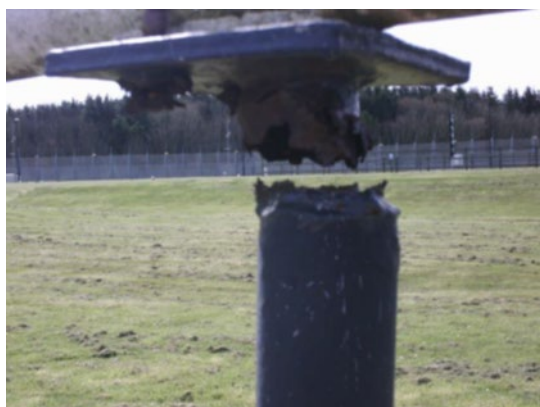
Figure 8: Damaged pipe support through corrosion and movement
