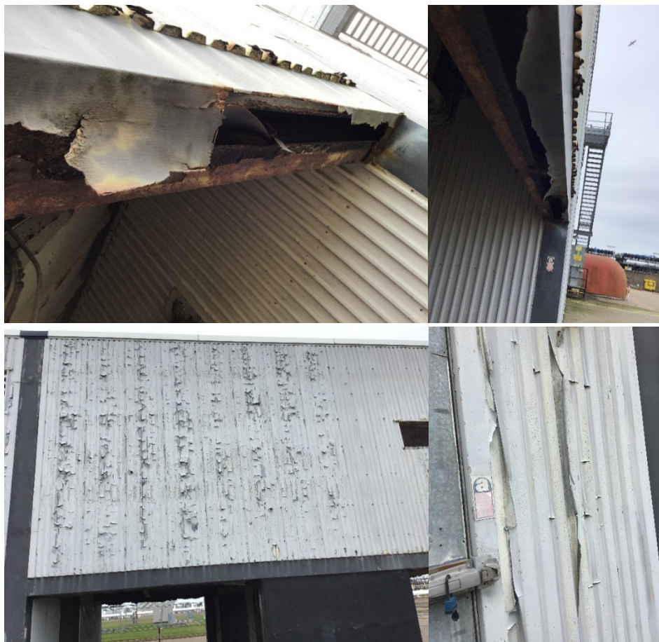
Figure 4: Coating breakdown of Galbestos cladding
