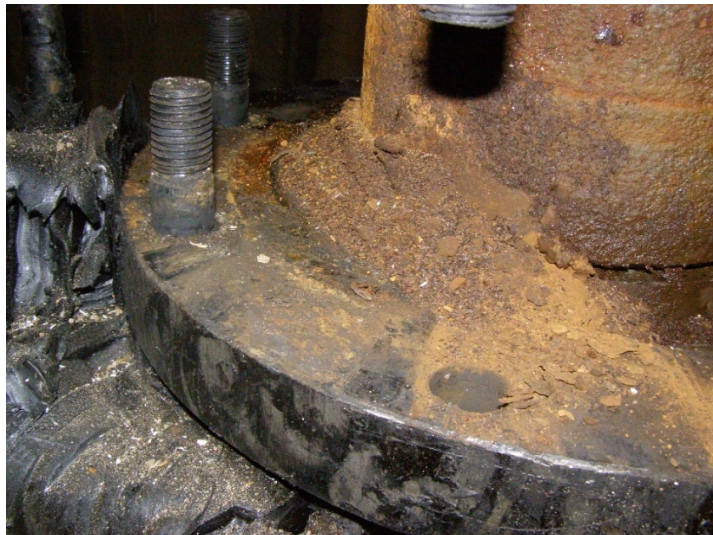
Figure 5 Debris and corrosion on the valve stem
