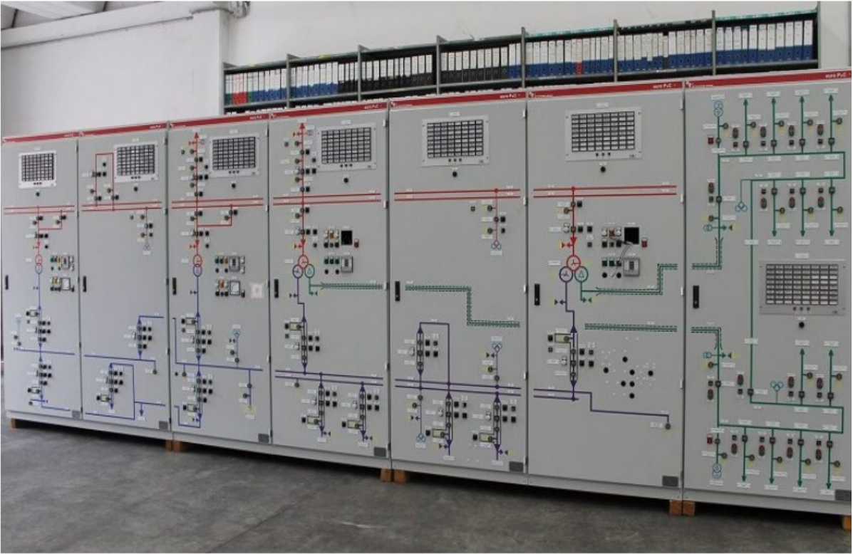
Figure 6: Typical compliant to best-practice standards switchboard
