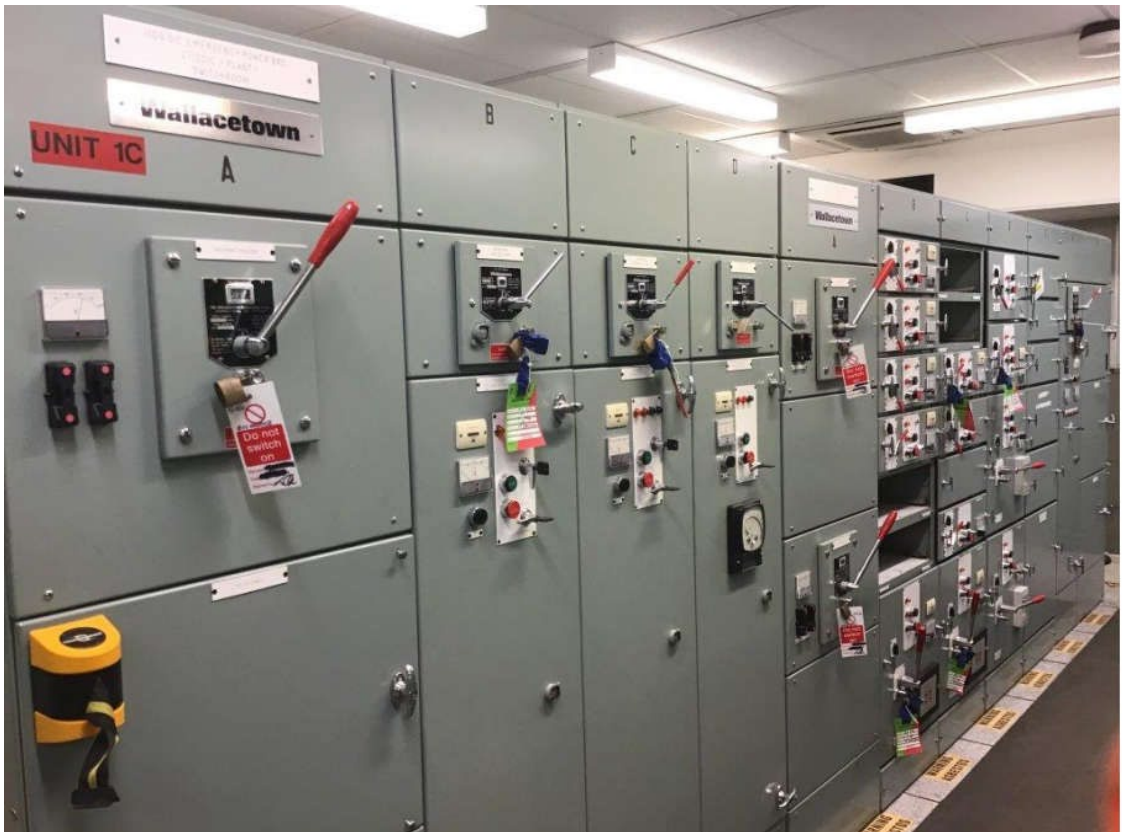
Figure 5: Compressor C1201C Switchboard G1
