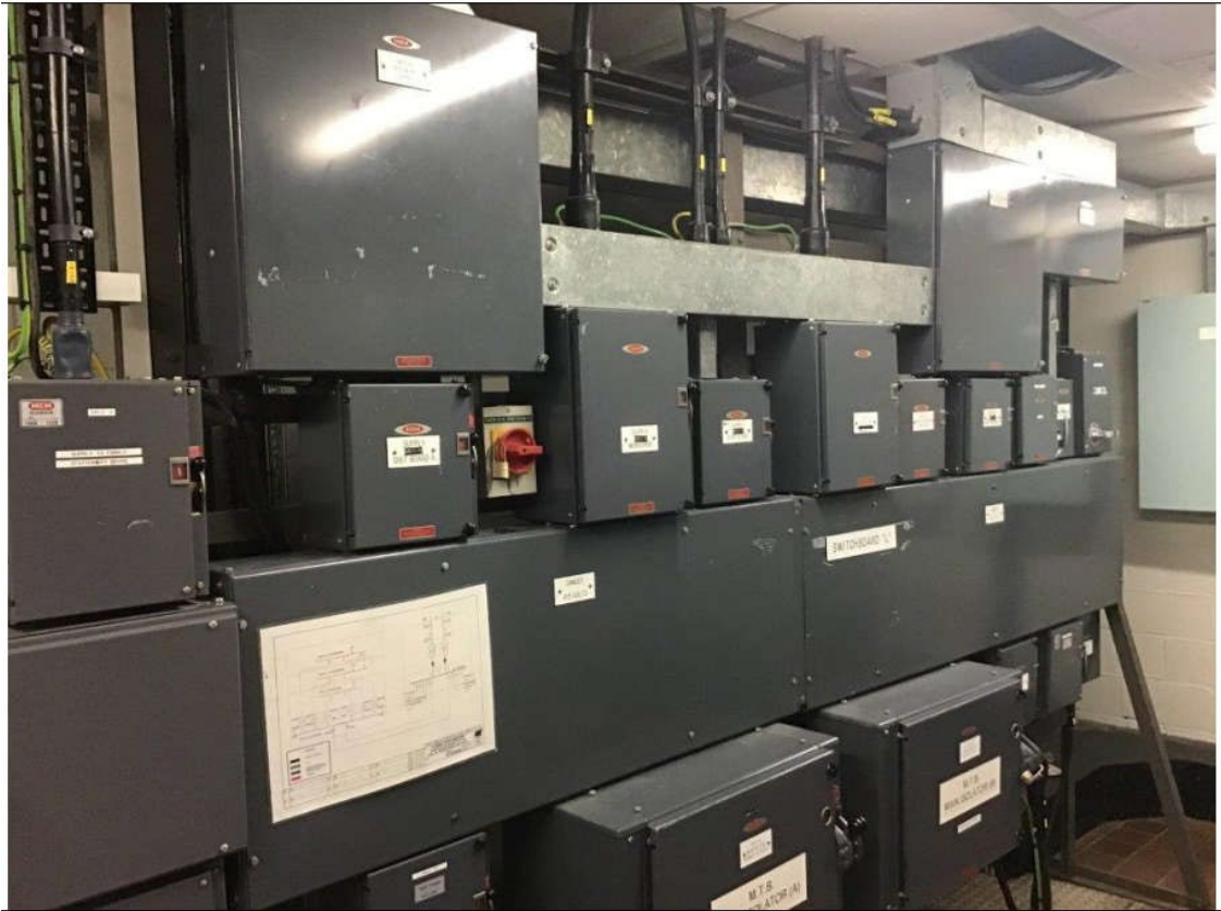
Figure 4: Building Services Switchboard 'L'
