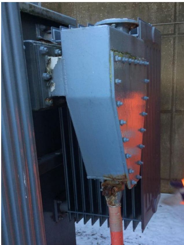
Figure 8 Corrosion on the radiator fins and connecting cables
