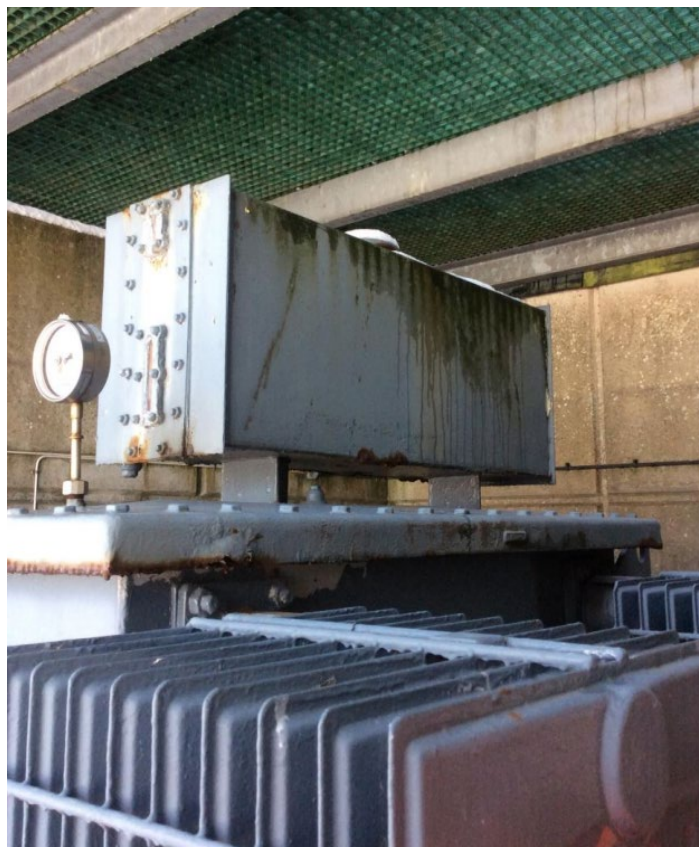
Figure 9 Leaking oil from conservator tank and corrosion
