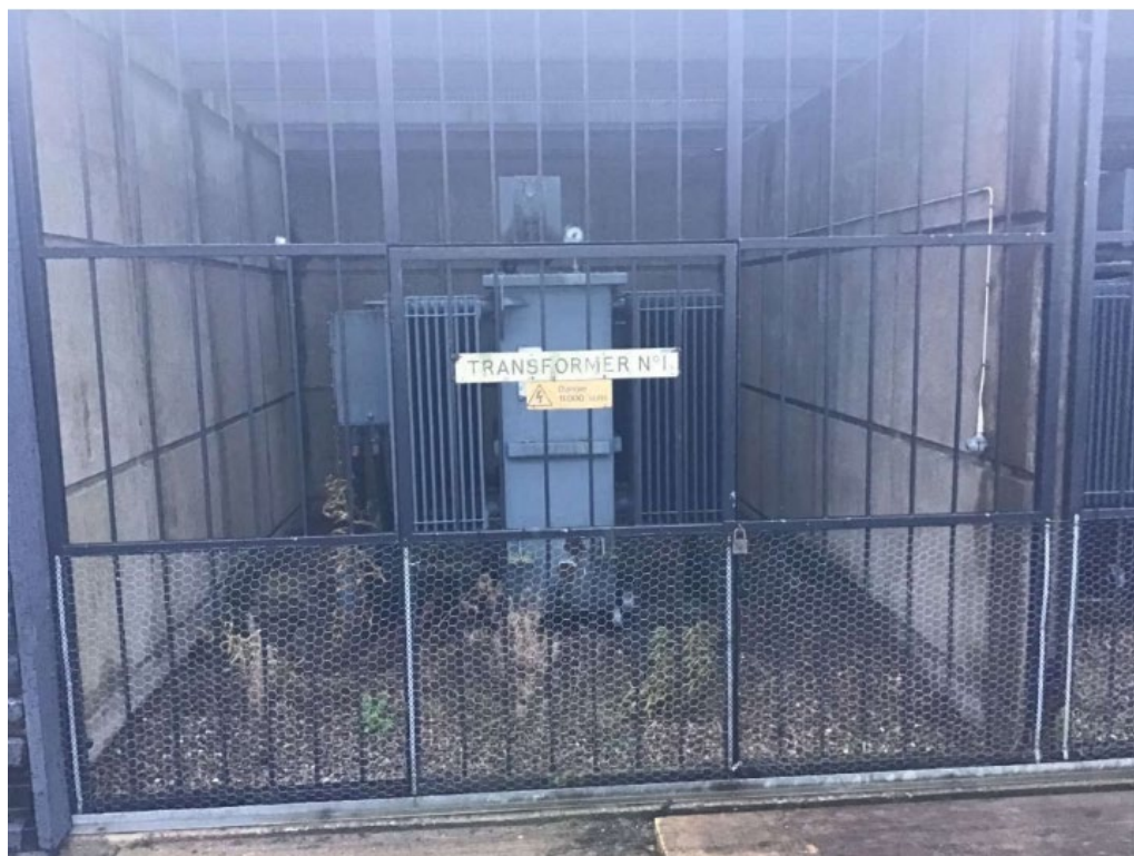
Figure 7 Plant 1 T1 transformer 1 currently isolated
