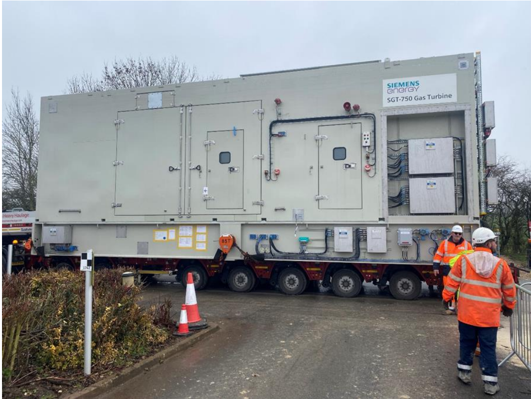
Figure 32 – SGT-750 Gas Turbine package being delivered in March 2023
