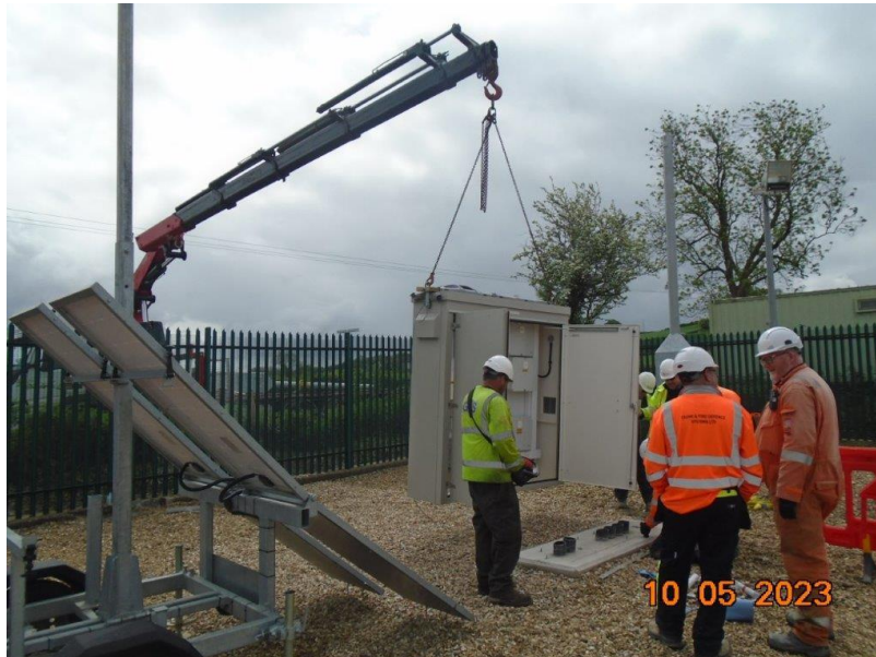
Figure 64 - Installation of control cabinet pre-built off site to reduce on-site working time
