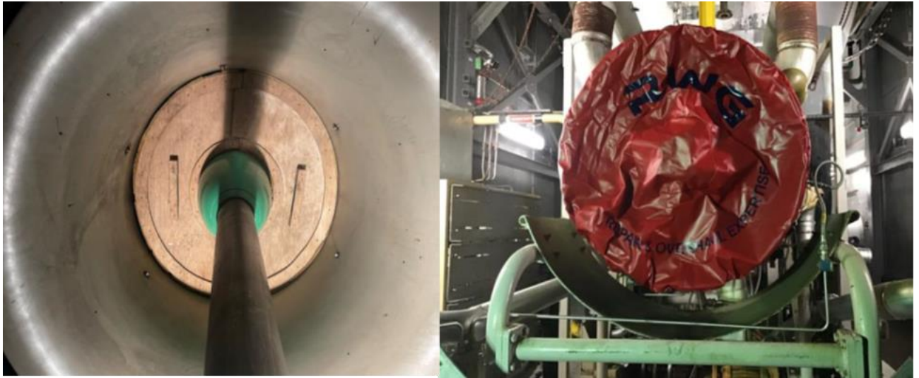
Figure 13 - Compressor which has been removed for engine inhibiting
