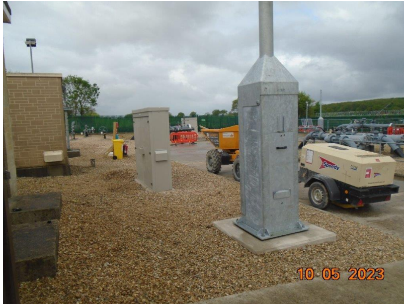
Figure 63 - New security tower and cabinet at Barrington AGI
