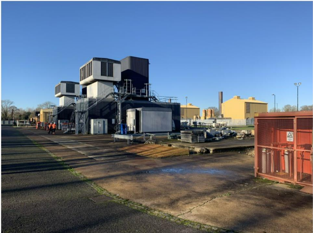
Figure 45 - Image of King's Lynn Compressors taken during site visit in 2022 - Avon Units A & B (black enclosures) front left with SGT-400 Unit D & E (cream enclosures) back right
