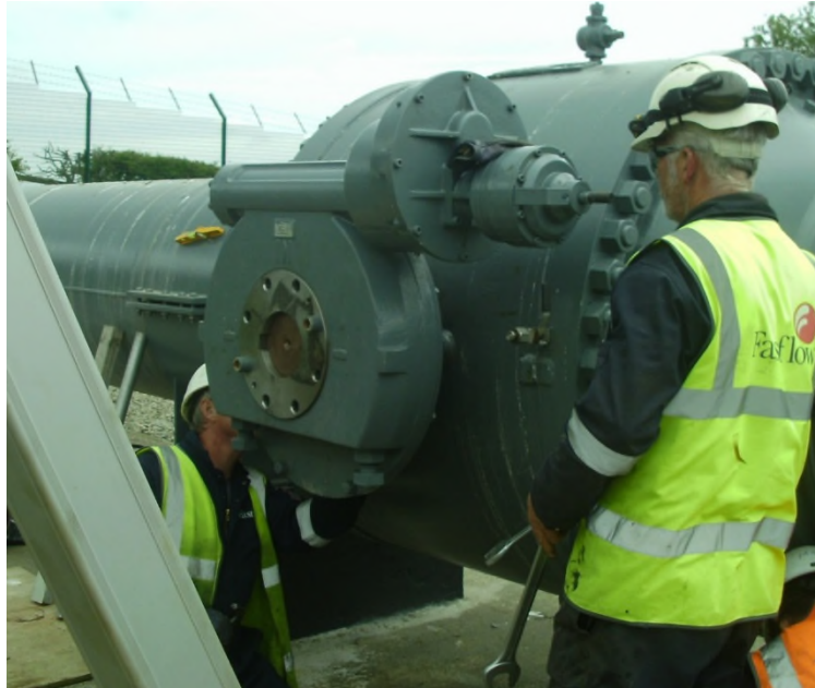
Figure 19: High Efficiency Gear Box installed
