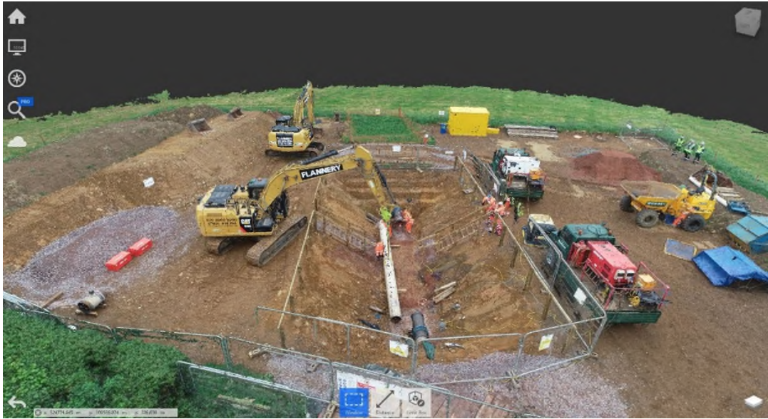
Figure 13: The Digital Rehearsal Plant Library was developed to improve efficiency and accuracy by the designer when developing the 3D rehearsal images and videos for buildability and safety assessments
