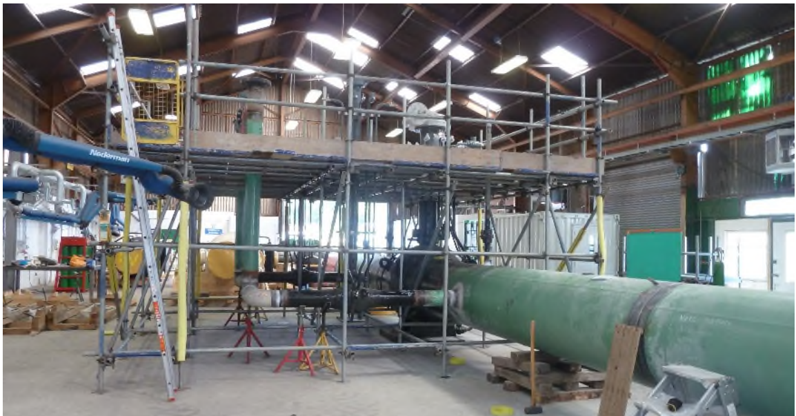
Figure 16 and 17: Overnight Installation of new Abernyte block valve (left), new Erpingham block valve installation (right)
