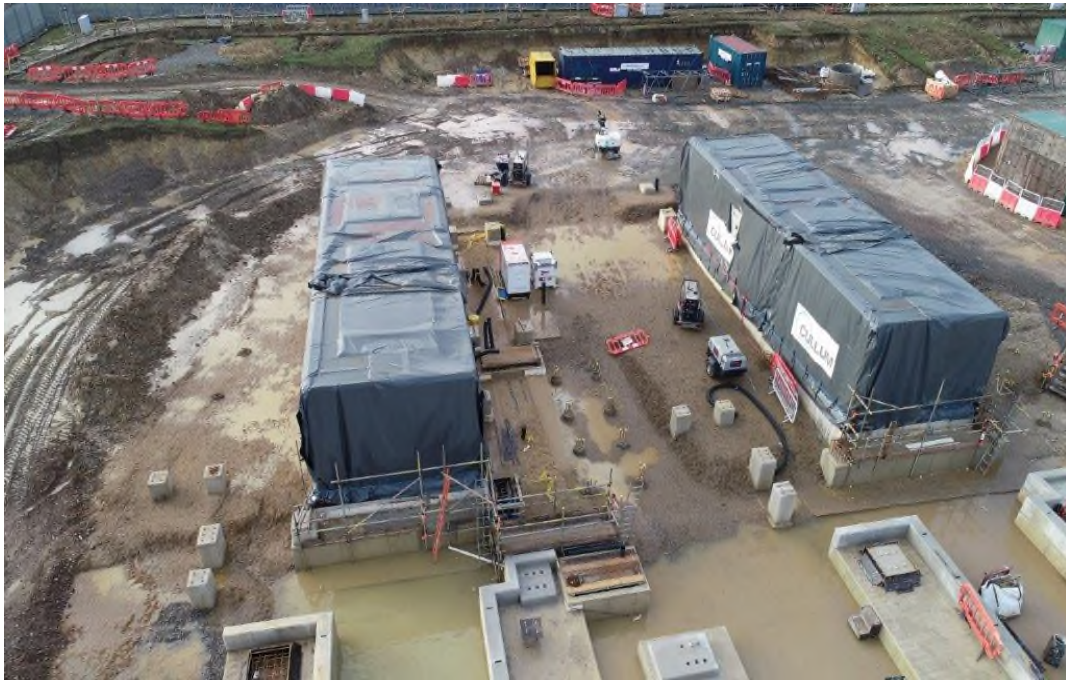
Figure 38: New Compressor Machinery Trains on bases at Huntingdon
