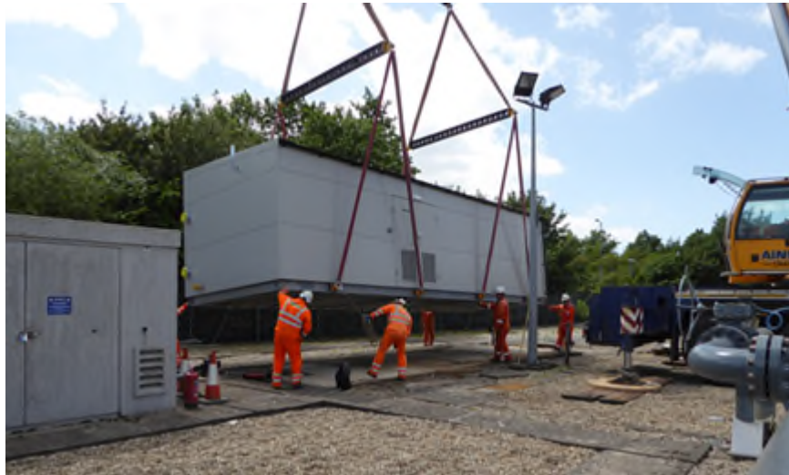
Figure 28 – The replacement boiler house being delivered onto the existing base at Kings Lynn
