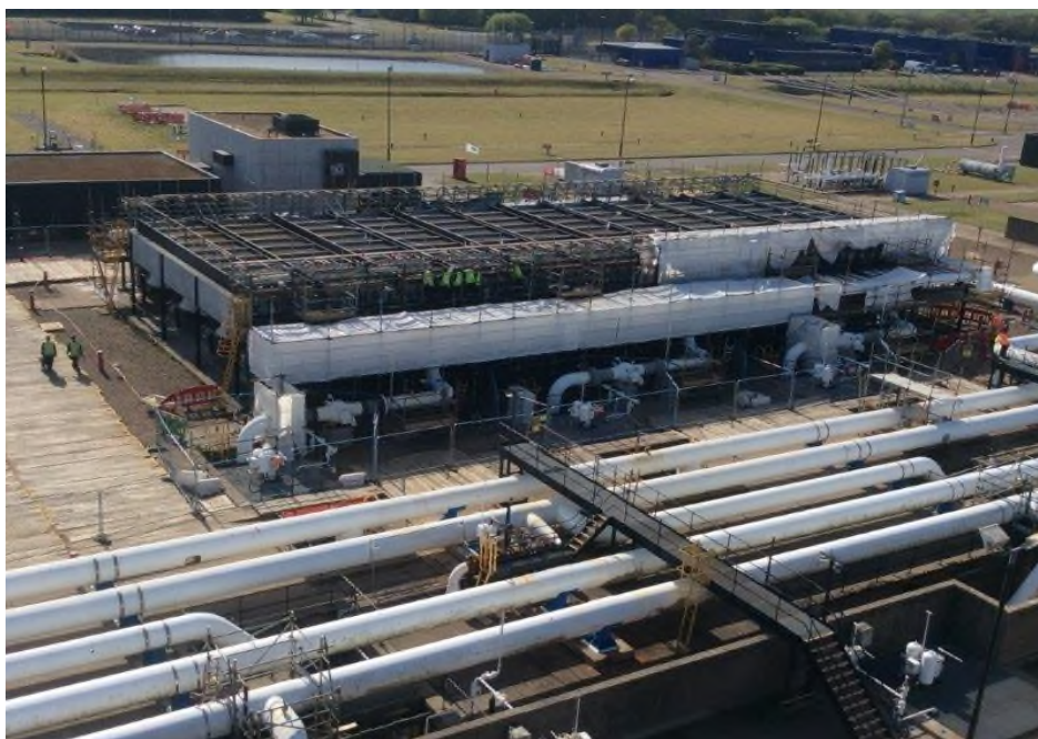
Figure 23 - Revalidation of 'Fin Fan' tubes and corrosion remedial works at St Fergus Plant 1 Aftercoolers
