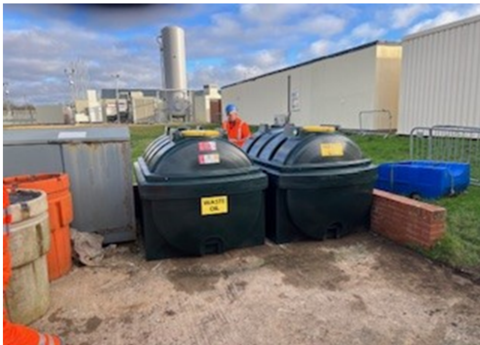
Figure 42 – New tanks installed at Peterborough AGI
