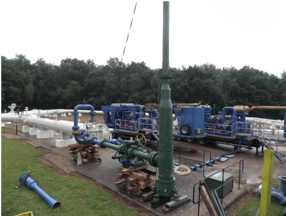
Figure 15 - Recompressor unit with the temporary vent stack (green) on site at a multi-junction on the NTS
