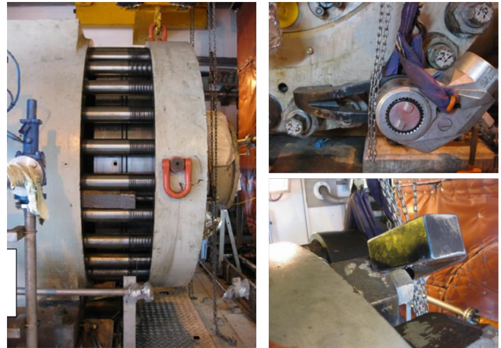
Figure 48 – New compressor assembly being installed at Aberdeen Unit A following dry gas seal change.
