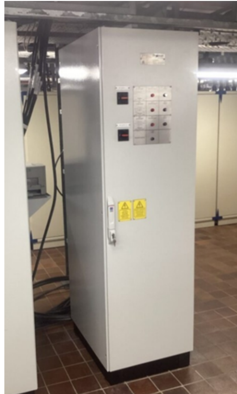
Figure 55 - New SIS control panel installed in Bacton switch room
