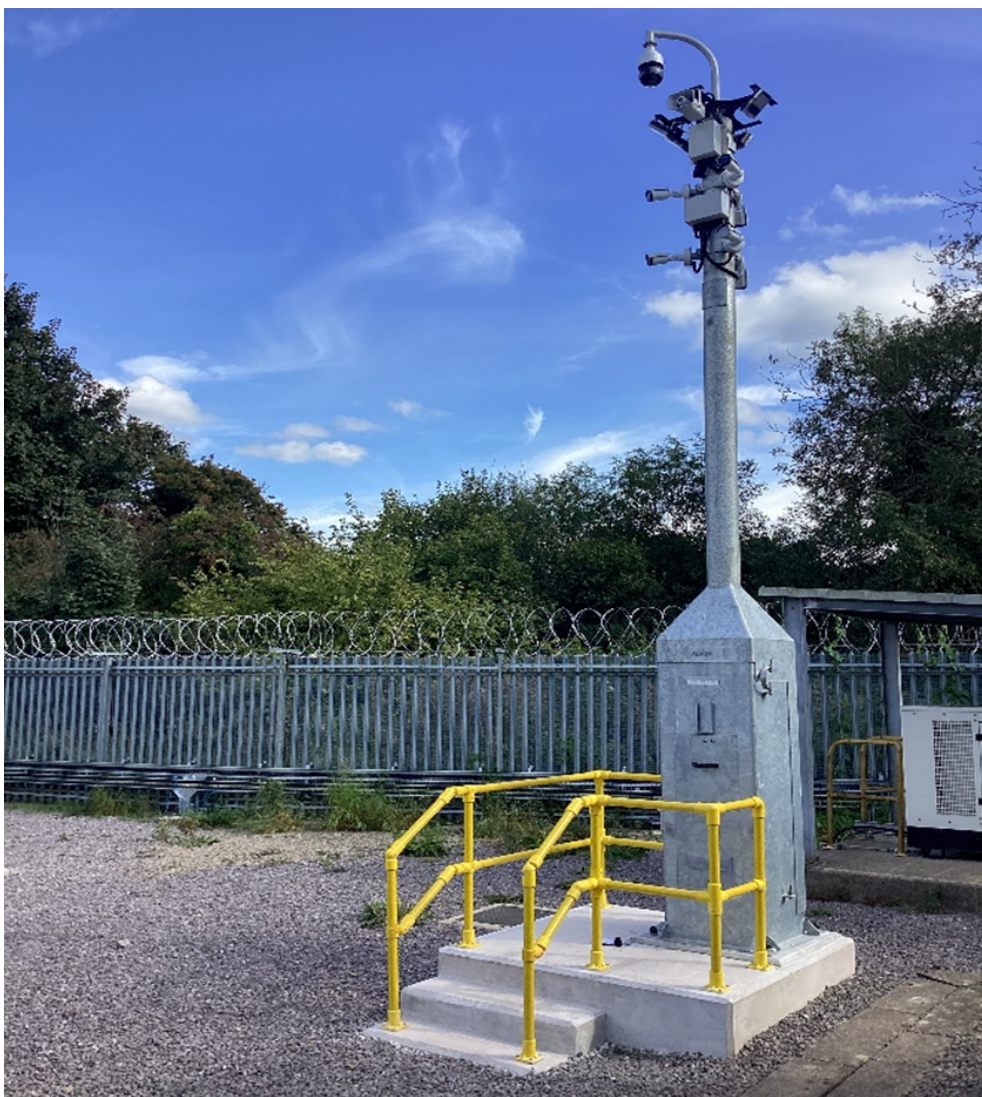
Figure 61 – Security tower with access platform comprising of CCTV, thermal cameras, audio challenge speakers and infrared and white lighting
