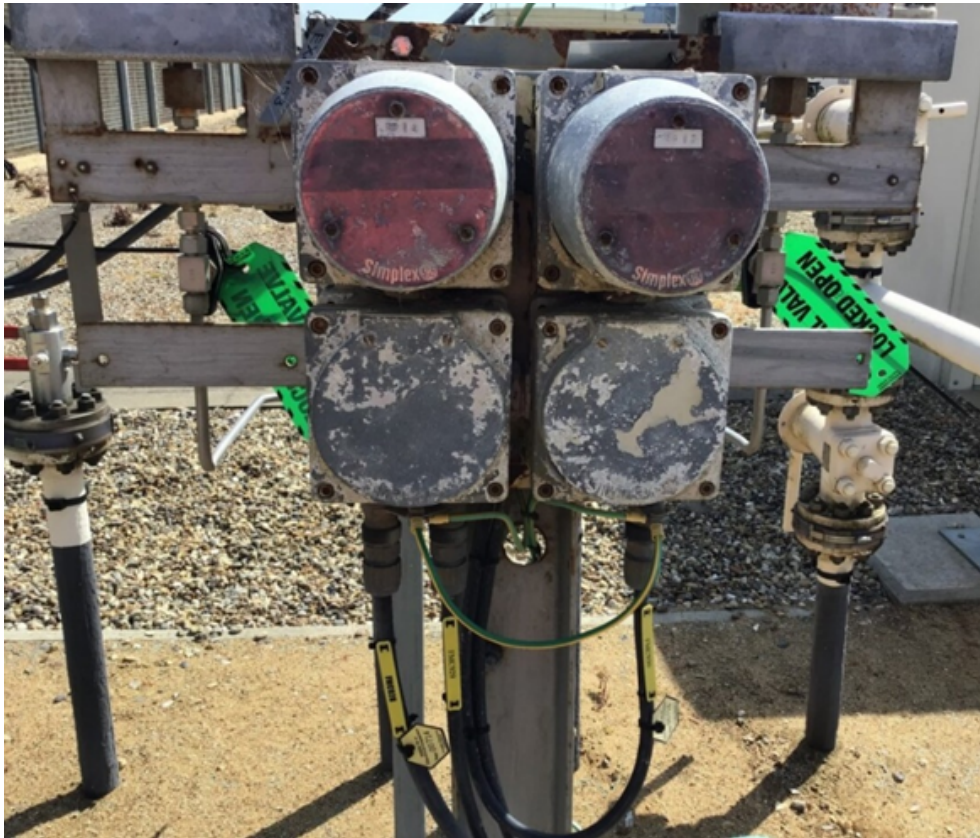
Figure 54 - Original control relays for Perenco 1 and 2 incomers. These have been replaced with a Safety Instrumental System (SIS) panel and Safety Logic System (SLS)
