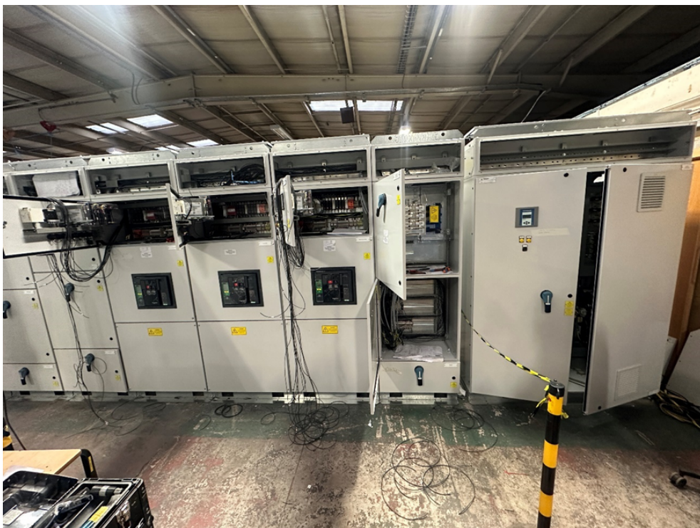
Figure 51 - Switchgear being fabricated for delivery and installation summer 2024
