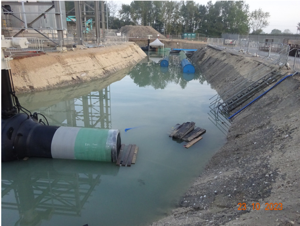
Figure 29 - Flooding from bad weather in October 2023
