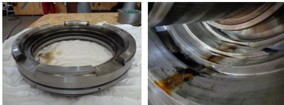
Figure 47 – Liquid identified when removing barrier seal. Seal gland cleaned prior to the installation of a new barrier seal.
