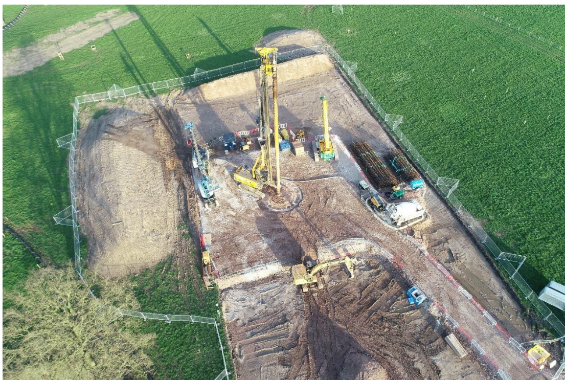
Figure 44: Aerial view of site establishment and commencement of reception shaft works on HS2 crossing.
