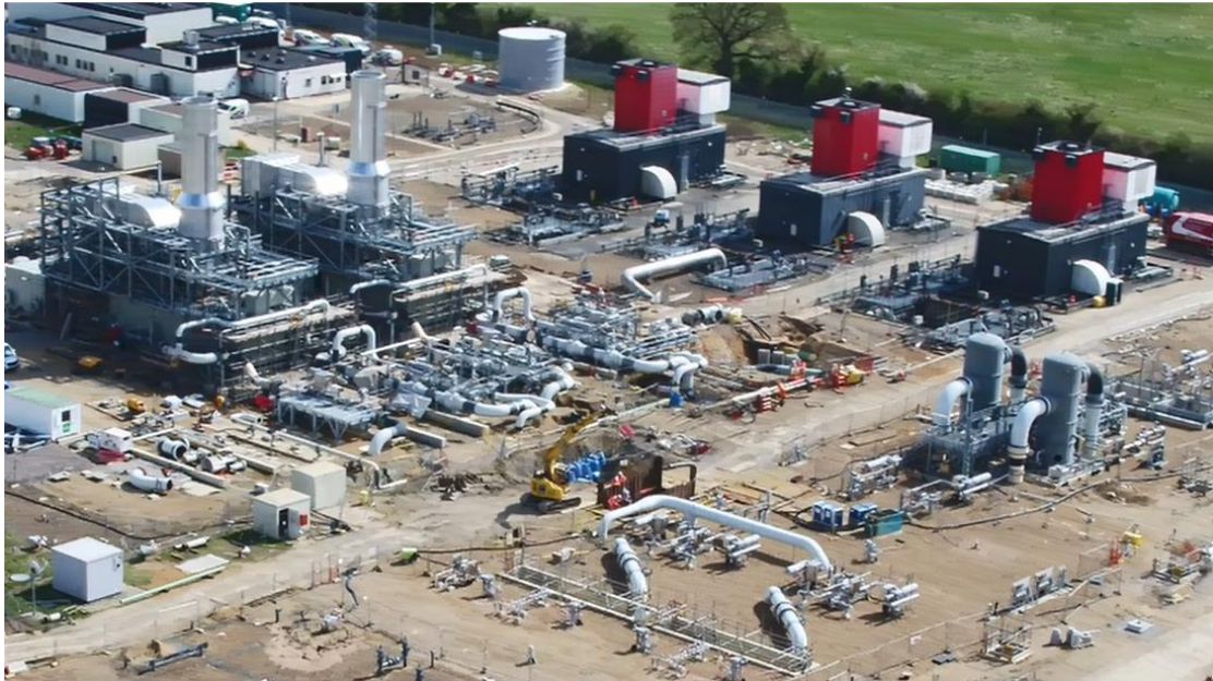
Figure 22: Image of the ongoing construction works at Peterborough. New units D and E are shown (left) with existing Avon units A, B and C (right)
