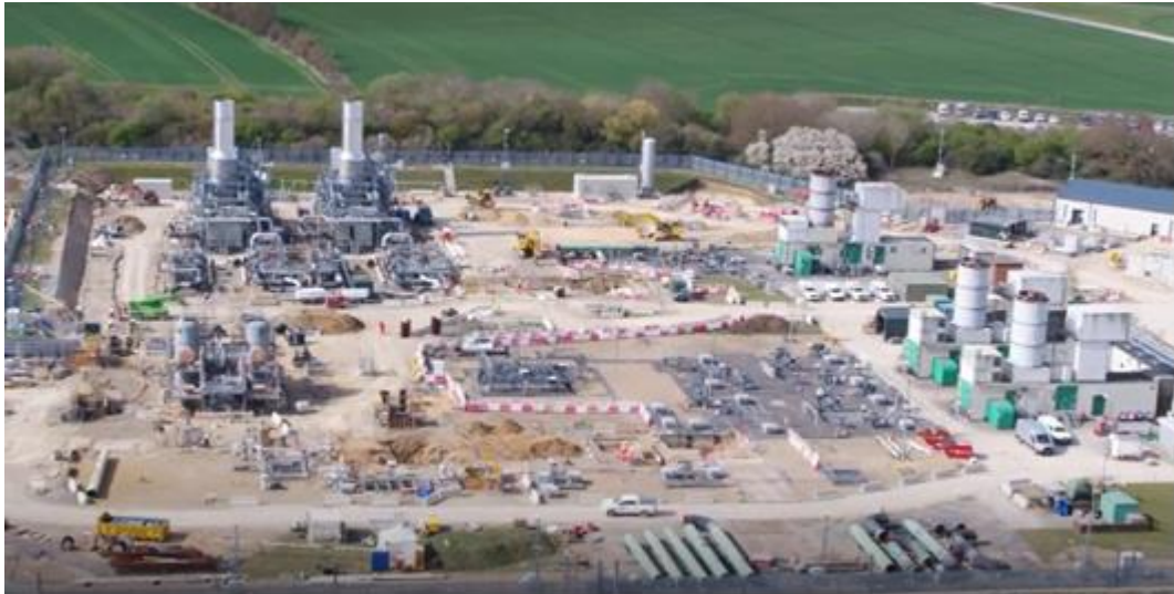
Figure 20: Image of Huntingdon showing installation works associated with two new gas driven compressors (top left) with existing Avon units (right)
