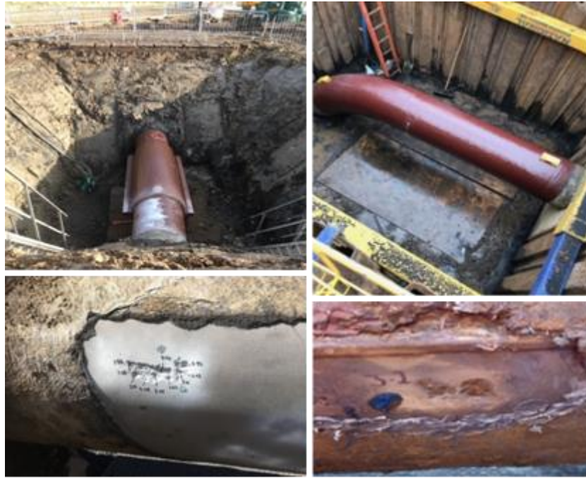
Figure 37: Examples of some of the 2021/22 pipeline corrosion defects and rectifications
