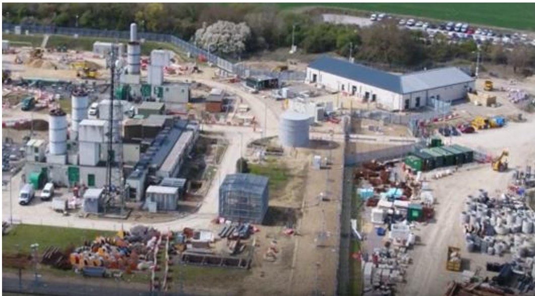
Figure 21: Image of from Huntingdon showing installation of new Control Station (top right); existing Avons can be seen (left)
