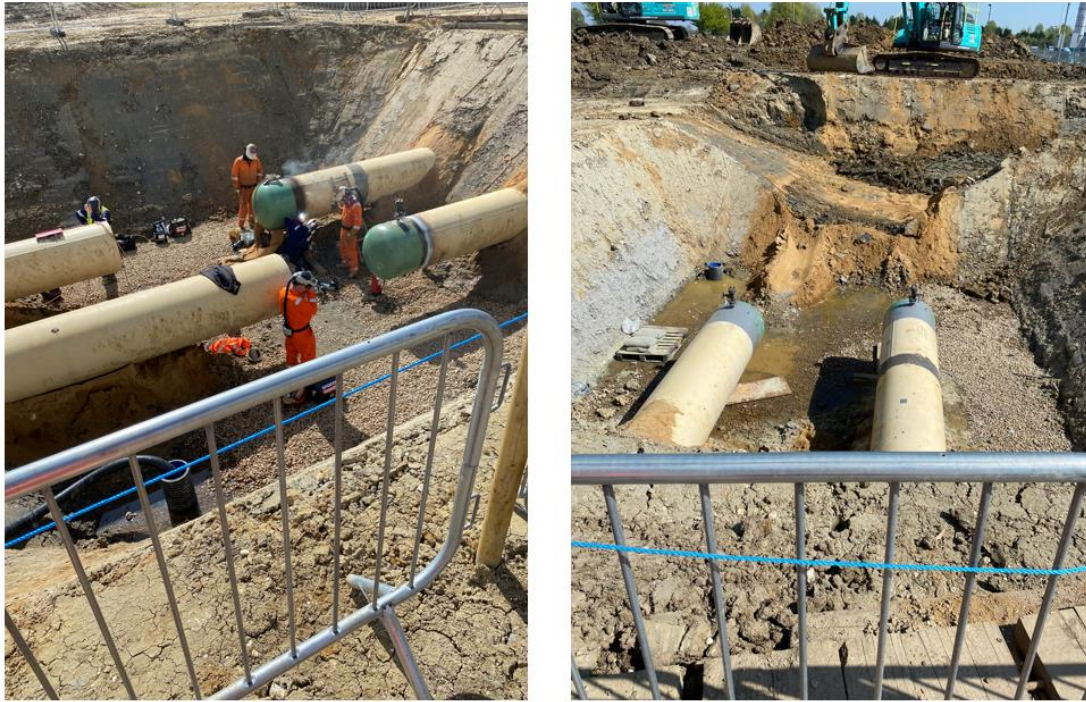
Figure 24 and 25: Hatton construction works - Cut, cap and removal of redundant 36" pipe between AGI and Compressor station
