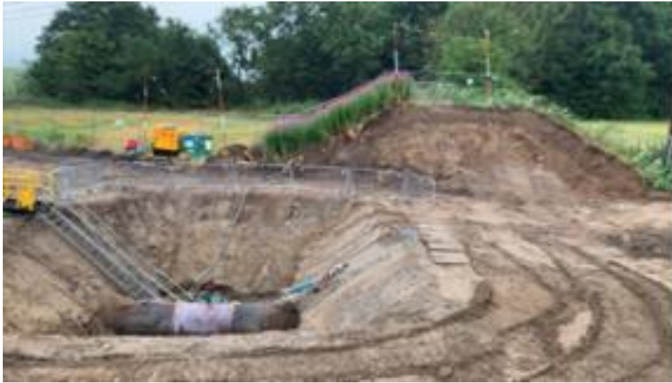
Figure 38: Groundwork to remove seven meters of ground cover and redundant railway banking
