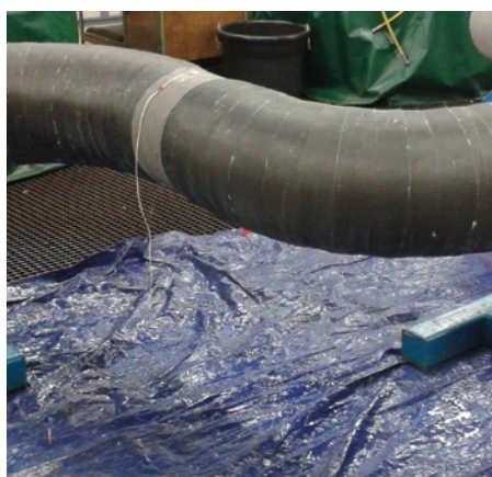
Two back-to-back bends with composite repairs applied over simulated corrosion patches, in preparation for fatigue testing.
