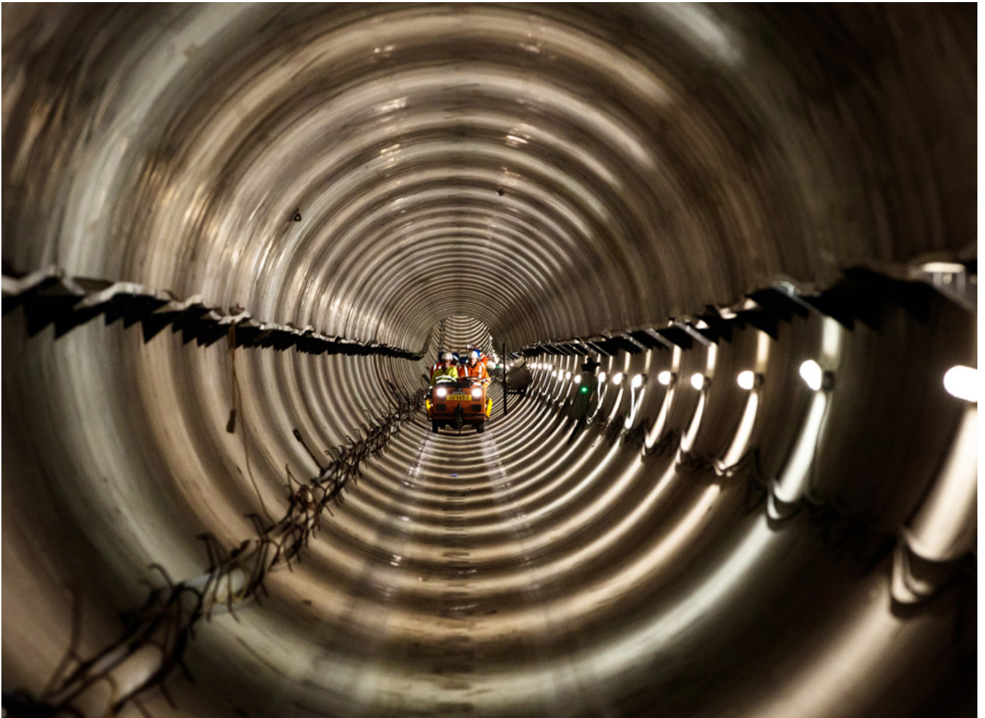
The 'Hidden Hero' - the Humber Pipeline Tunnel enabling a crucial feeder pipe to supply up to 20 percent of annual gas supplies to the South of England
