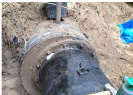
Figure 8: Defective Nitrogen Sleeve End Seal
