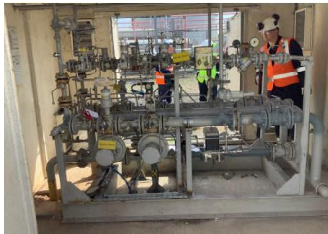
Figure 15: [REDACTED] Preheating Fuel Gas Regulator Skid
