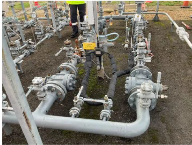
Figure 16: [REDACTED] Main Pressure Reduction Skid
