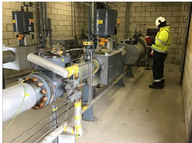
Figure 12: [REDACTED] Pressure Control Valves.
