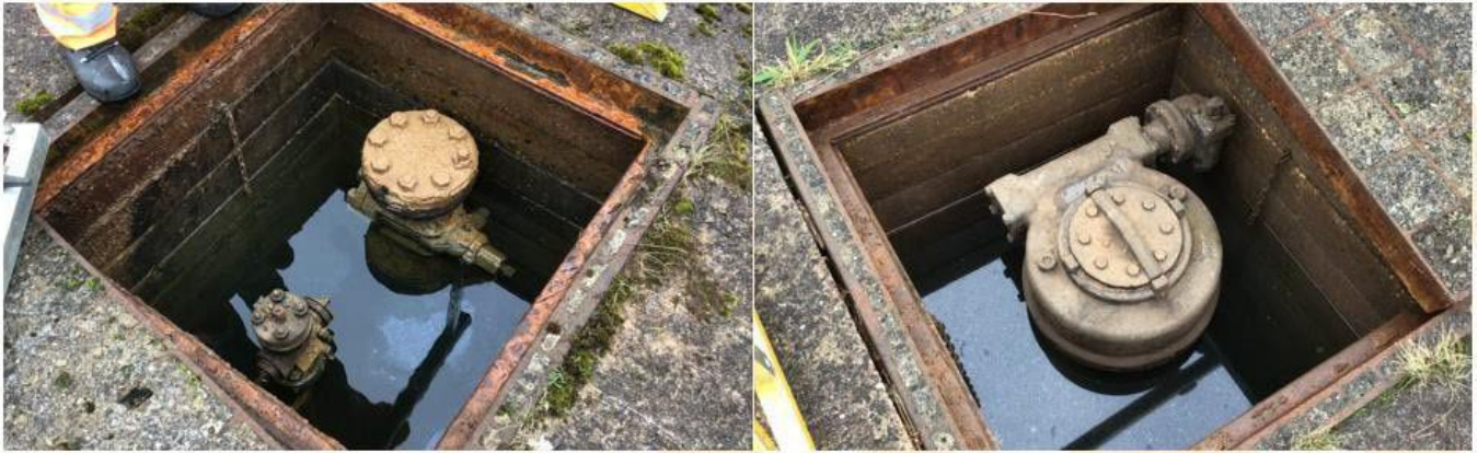
Figure 3: Insufficiently sized pit for valve maintainability
