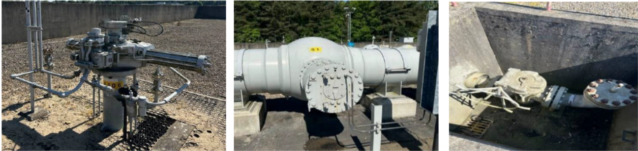
Figure 1: Below ground valve and its above ground operator, above ground valve and a valve in a pit.
