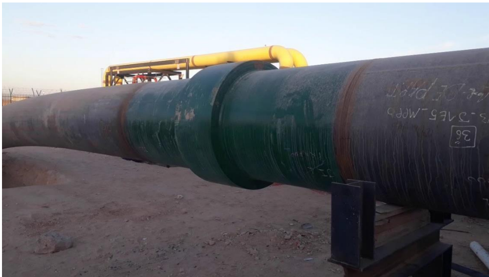
Figure 11: Insulation Joint on a above ground pipeline (Not NGT asset)
