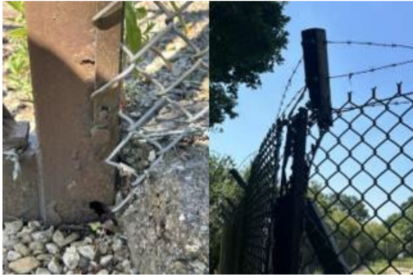
Figure 6: Corroded gate and fence posts at [REDACTED]
