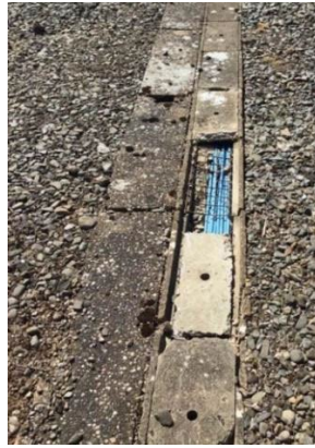
Figure 22: Broken ducting [REDACTED]
