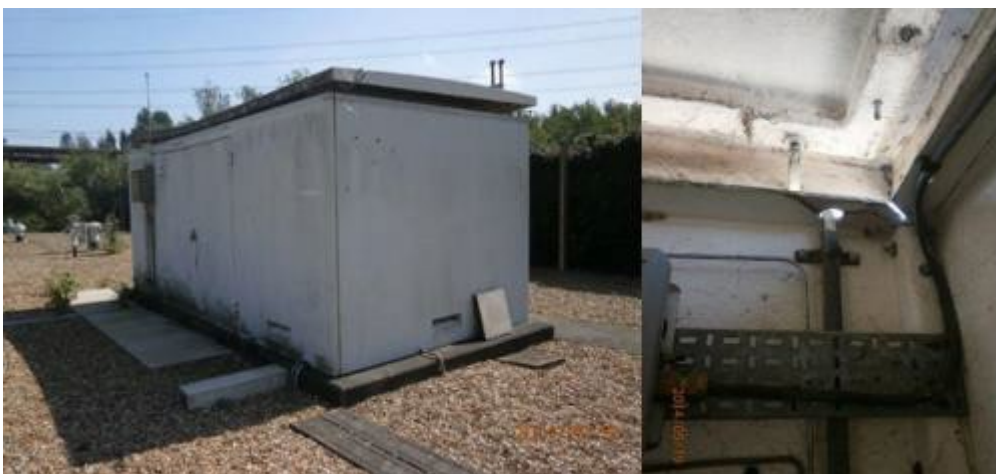
Figure 5: Damaged roof of enclosure [REDACTED]
