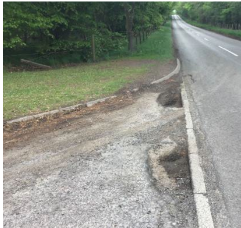
Figure 20: Potholes on access road [REDACTED]
