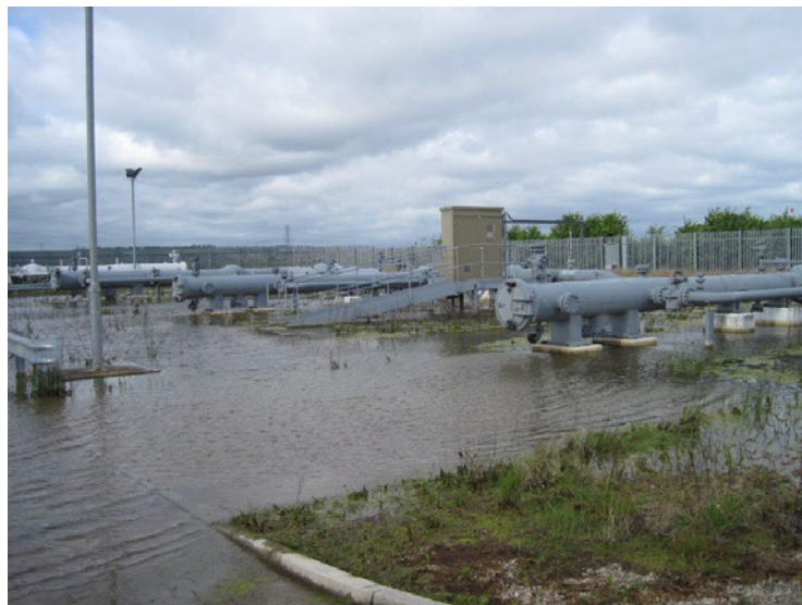
Figure 9: Flooding at [REDACTED]
