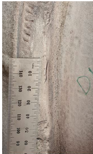
Figure 3: Crack defect at [REDACTED] PIG Trap A
