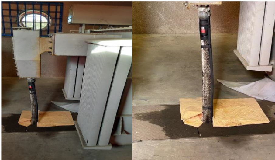
Figure 6: Bishop Auckland Transformer defects
