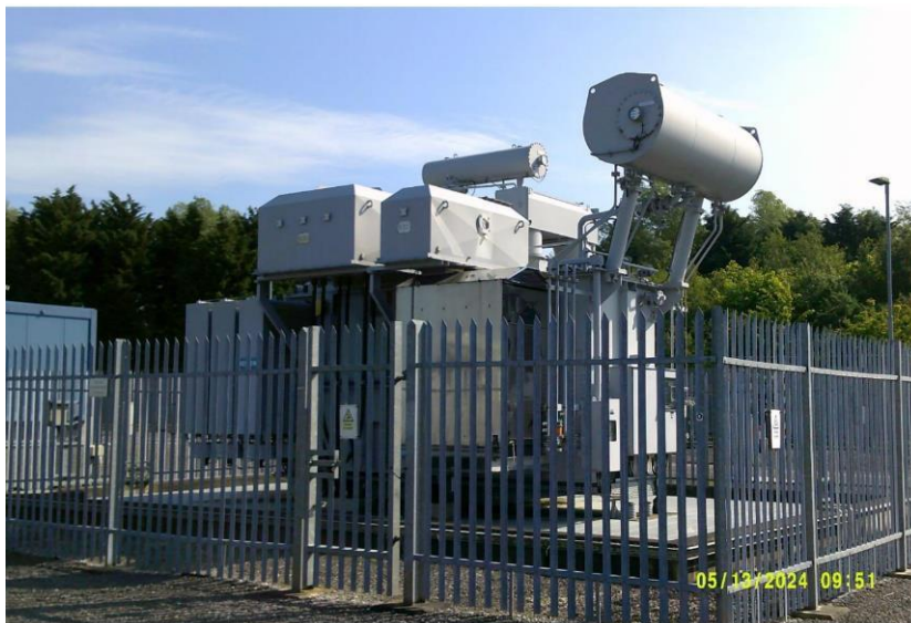
Figure 5: 132 kV to 33 kV distribution transformer utilised at [REDACTED]
