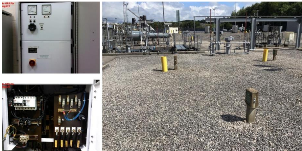
Figure 2: CP Transformer Rectifier and Test Posts (with reference electrode posts)
