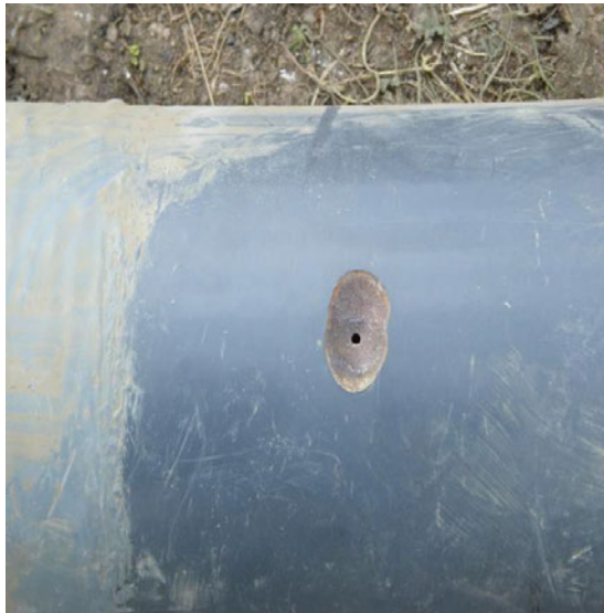
Figure 5: IP Gas Pipeline Through Wall Corrosion
