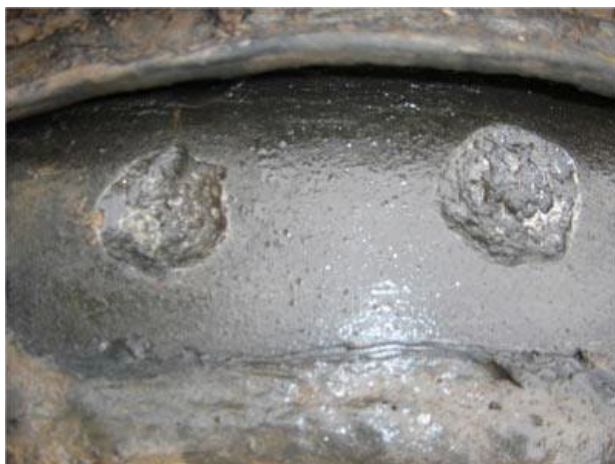
Figure 1: Typical AC Corrosion Feature
