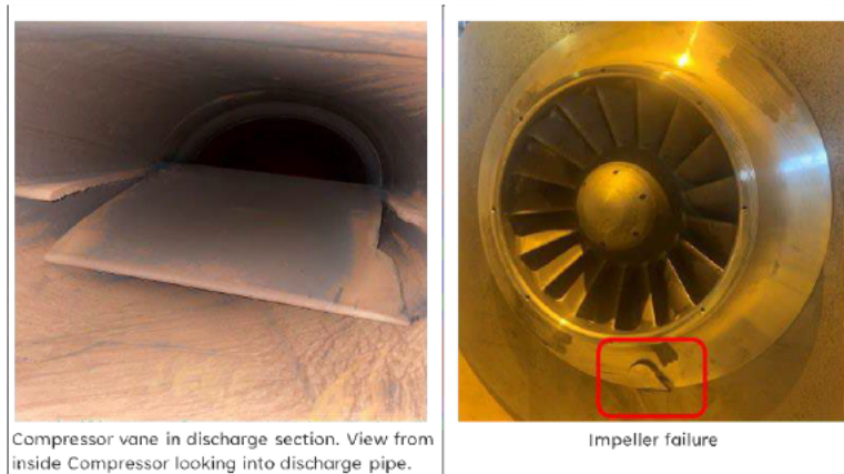
Figure 5: Cracked compressor vane and failed impeller.
