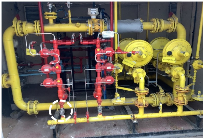
Figure 6 Stream A and B slamshuts (circled) with the bypass lines at [redacted]
