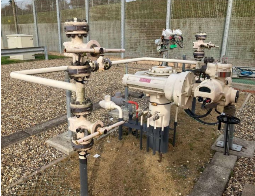
Figure 8 Example of safety valve with bypass installed [REDACTED]
