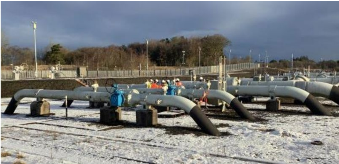
Figure 4 V15 Surrounding pipework arrangement [REDACTED]
