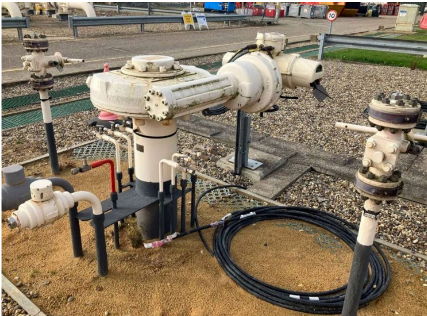
Figure 9 Example of safety valve without bypass installed [REDACTED]
