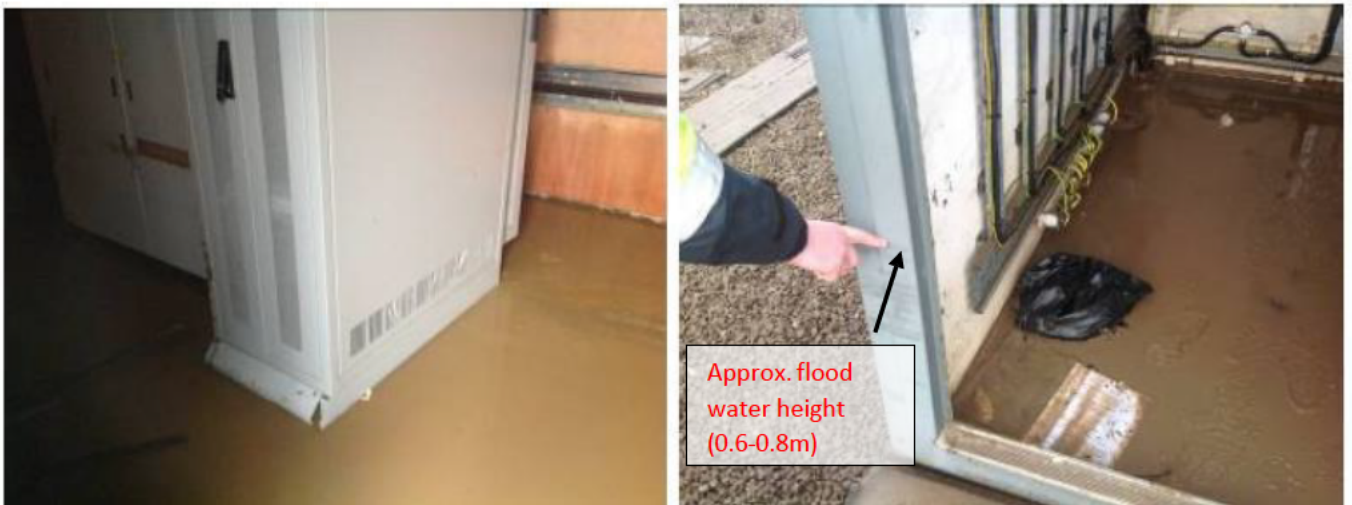
Figure 11: Internal and External Flood Damage, Flood-water Height in Most Places was between 0.6 to 0.8m
