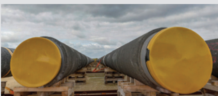
Pre-built pipeline sections for the pioneering Humber pipeline replacement, which will secure 20% of the country's gas supplies. Gas Transmission has engaged schools, local consumers, councils and voluntary groups to derive substantial community benefit from the project.
