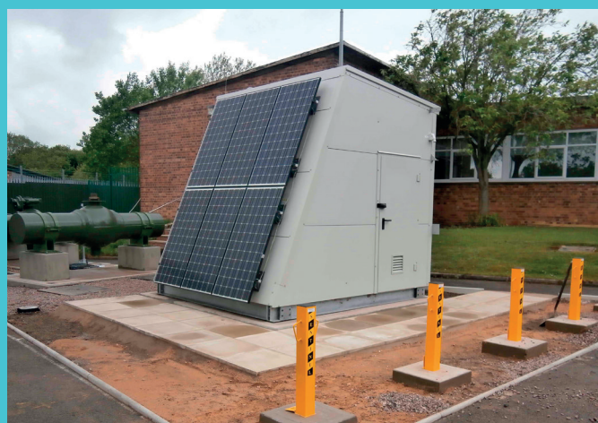
Renewable power kiosk
