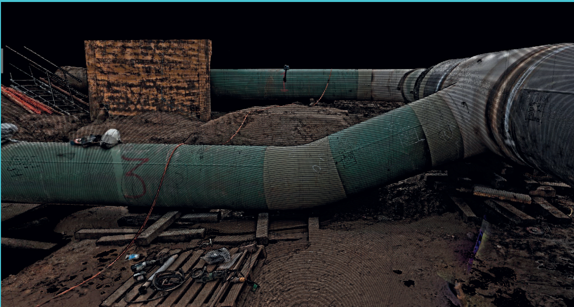
3D As Built – an example section of the laser-scanned pipework that will provide improved knowledge on the pipework after burial.
