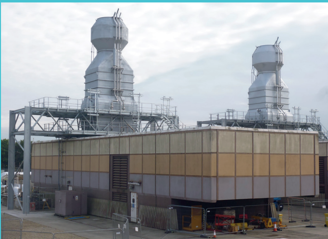
New exhaust stack and catalyst abatement system at Aylesbury compressor station.
