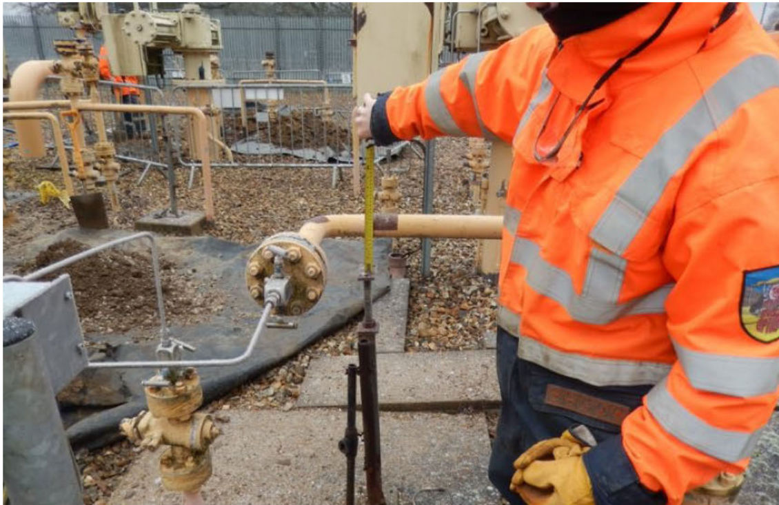
Photo 3 50NB pipe support subsidence compared to original height (Winter 18/19)
