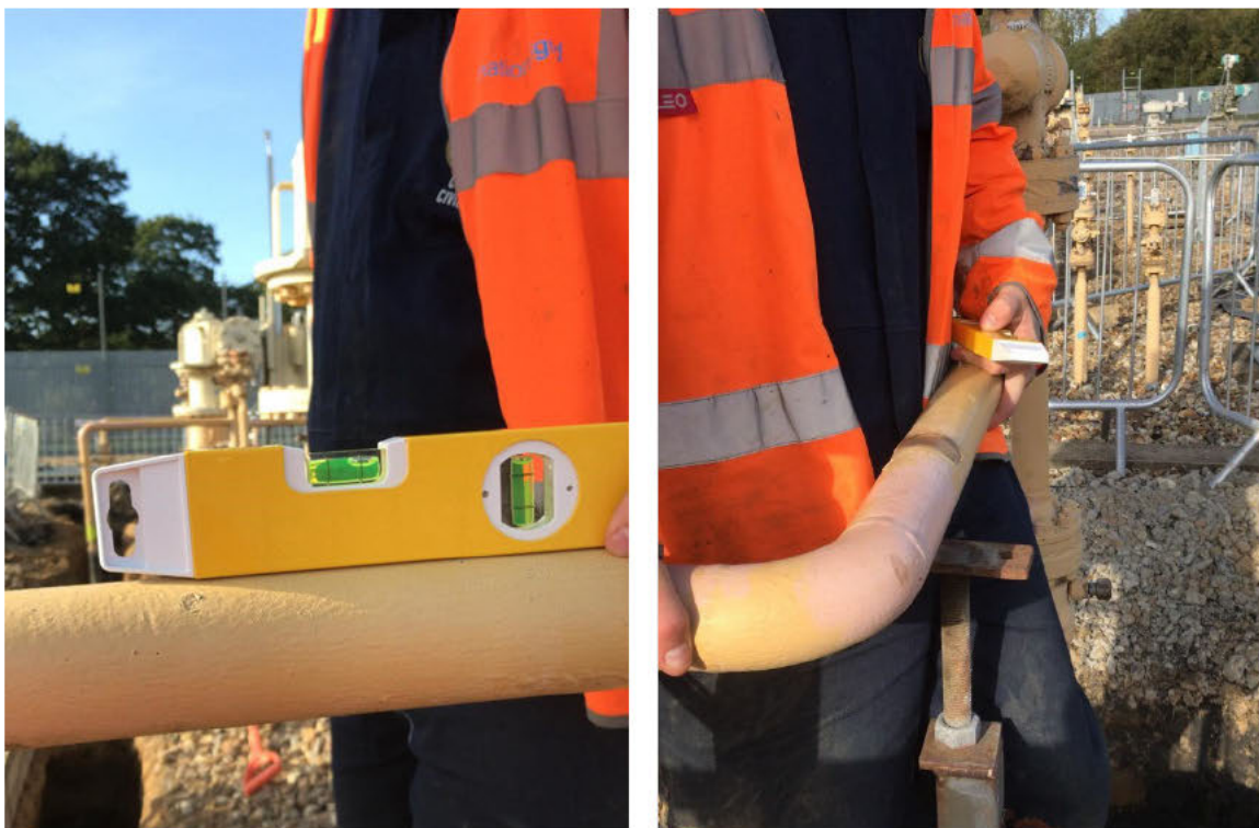
Photo 2 Evidence of subsided 50NB pipework and similar pipe support subsidence (Winter 18/19)
