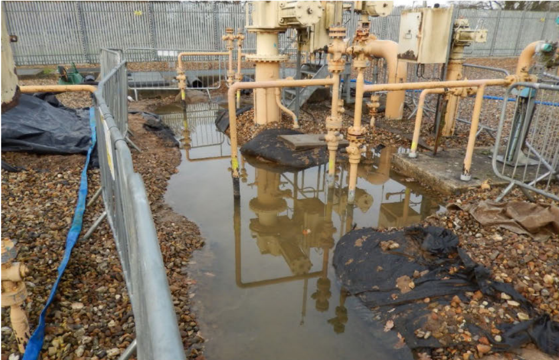
Photo 1 Water logging in part of bi-directional and evidence of 50NB pipe subsidence (Winter 18/19)
