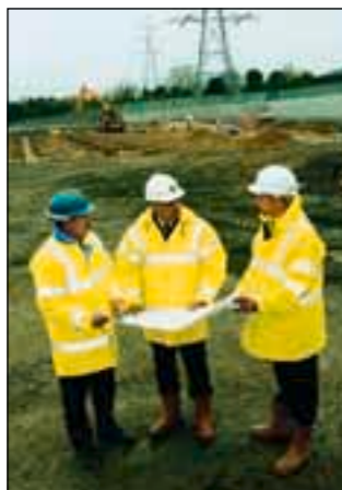
Back to the beginning... John Coughlin, with National Grid engineers' representative Russell Watkins and Howard Oley from VA TECH Reyrolle during the early days of the project
