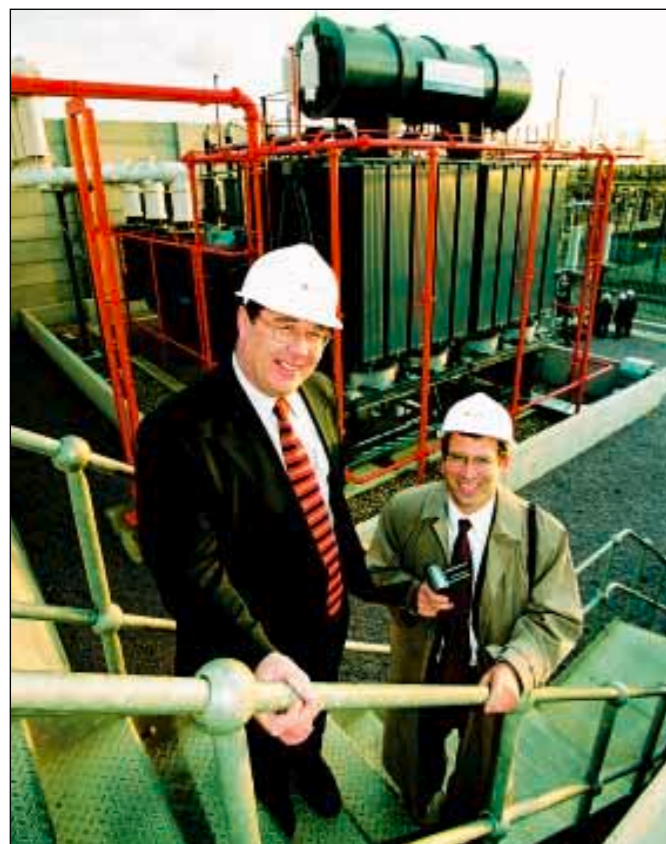
On site... NG substations manager Les Adams, left, and VA Tech managing director Charles Overstall
