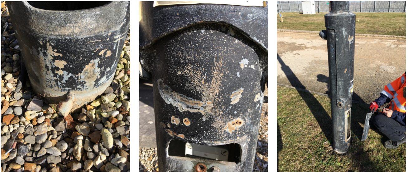
Corrosion of the column and reduction in the wall thickness particularly at the base of the column
