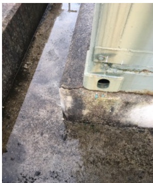
Corroded floor plate
