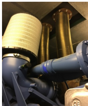
Heat detectors close to exhaust
