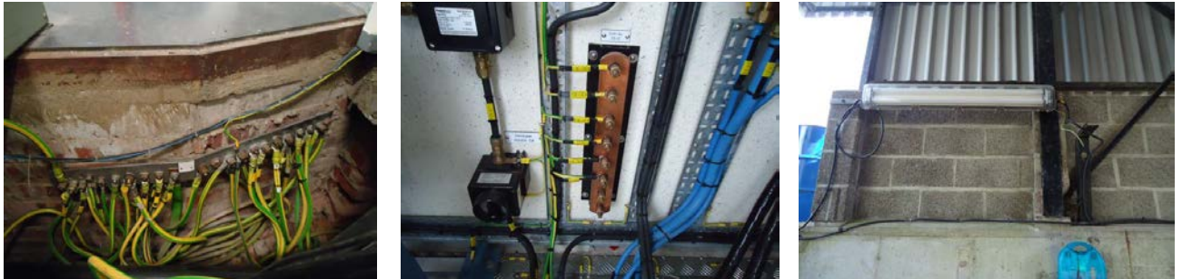
Degraded joints and broken earthing bonds
