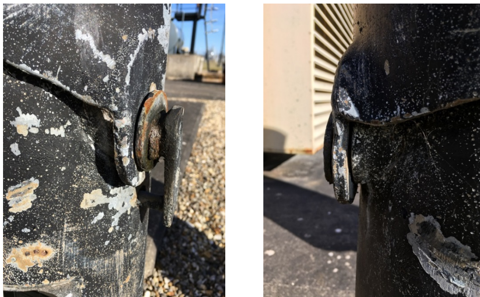
Corrosion of the hinge mechanism used to lower the column for maintenance.
