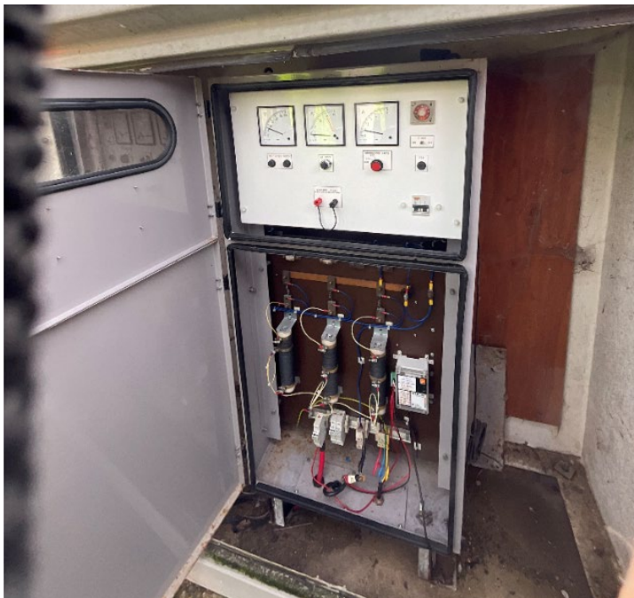
Figure 21 View inside a typical current TR cubicle
