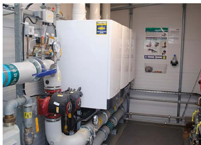
Modular boiler gas heating system on a HP reduction installation.
