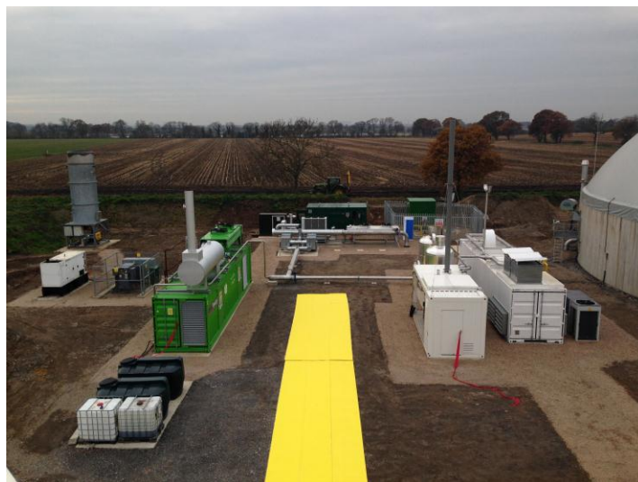
This is a picture of the Bio-methane facility that was connected to the National Grid Gas Distribution system at Lindholme, Doncaster in October 2013.
