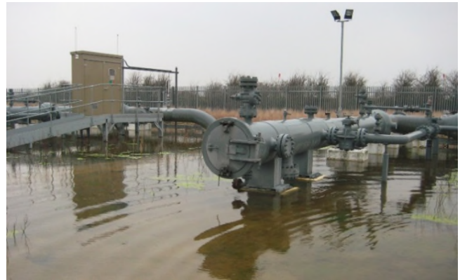
Figure 14.76 flooding at the Gravesend Thames South above ground installation in 2013
