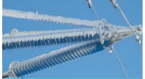
Ice build up on crossarm
