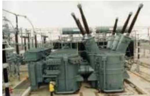
Transformer Life Management Improvements
